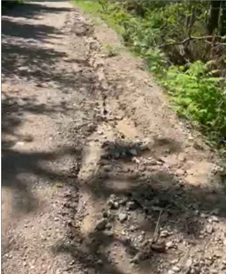
Site Photo 1: Existing Driveway Erosion
