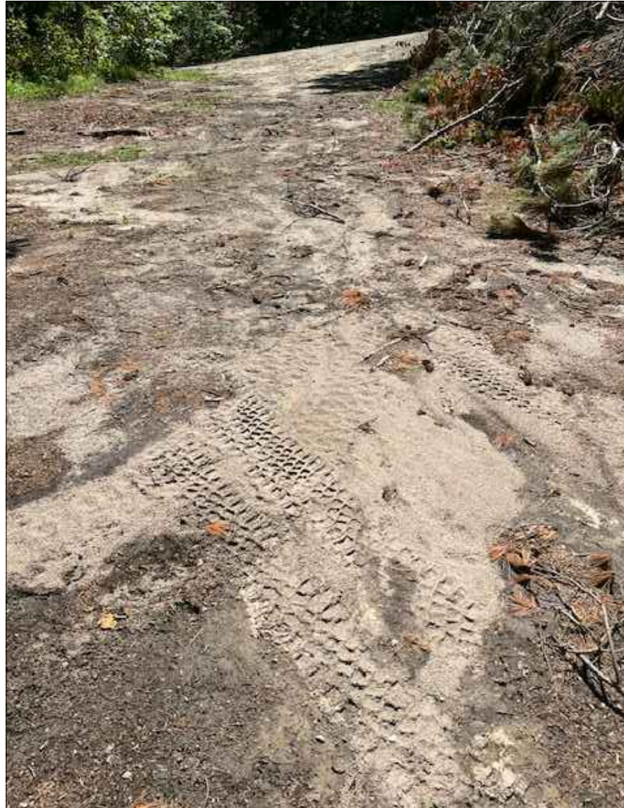
Site Photo 2: Sediment Caused by Erosion
